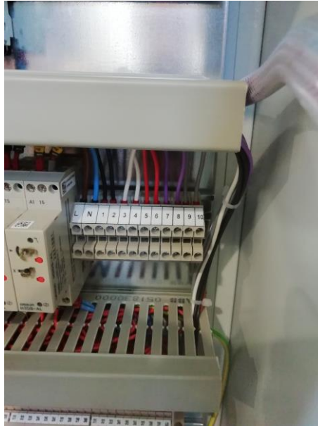
Terminal box condenser unit generator
