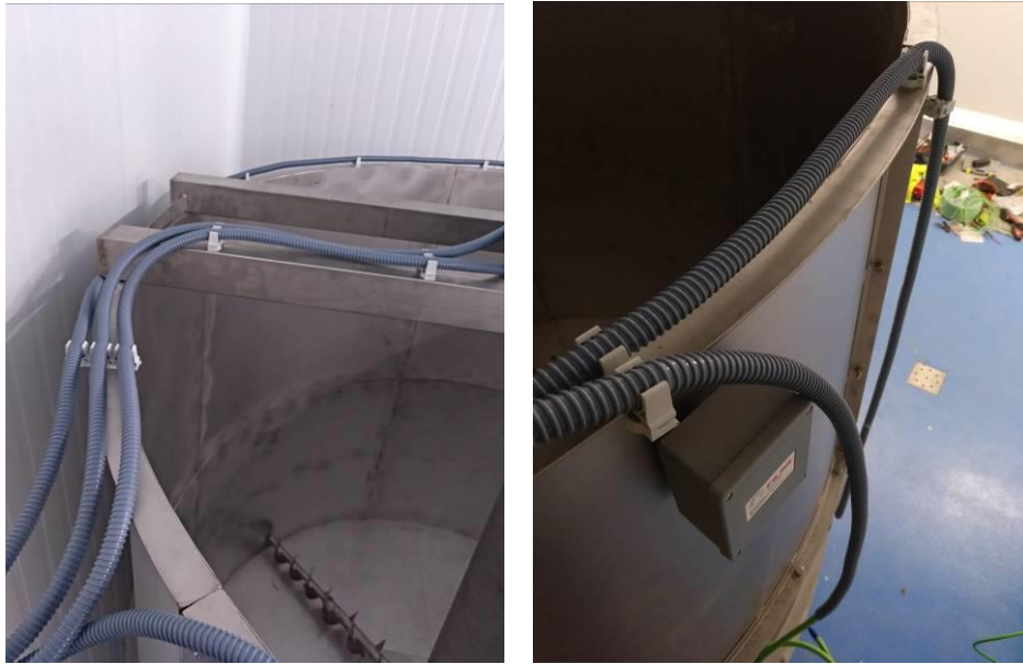
Wiring on the top of the bin
