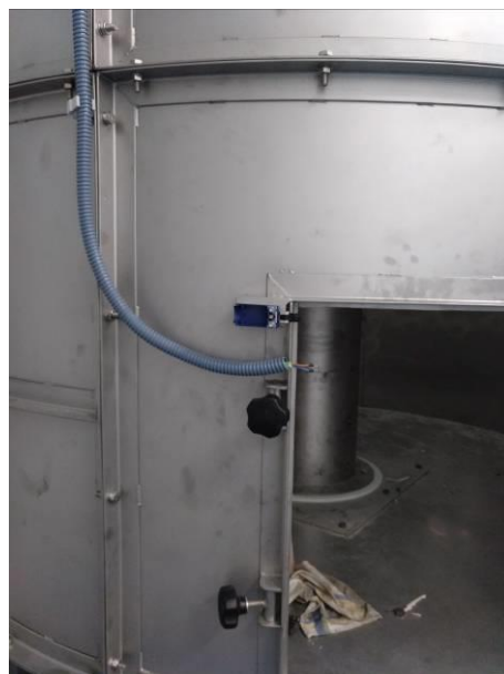
Door opening safety relay
