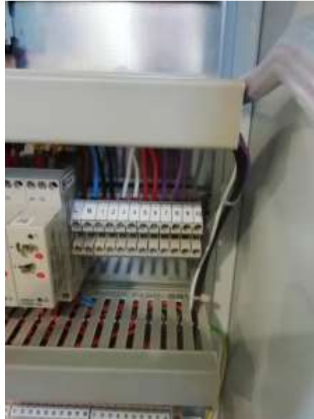
Terminal box condenser unit generator
